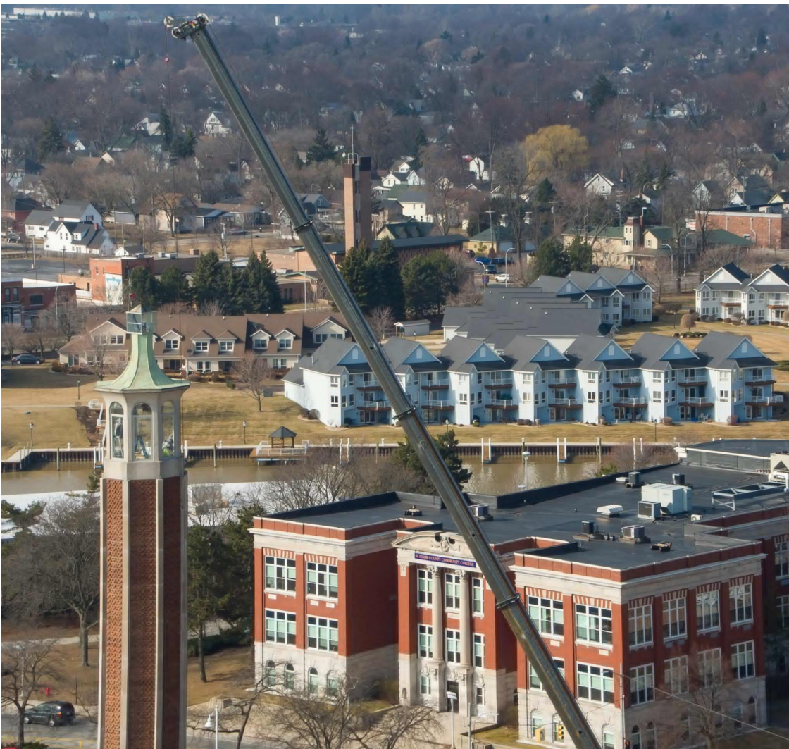
New windows are being installed on the @[131054075632:274:St. Clair County Community College] tower. Glad to see them investing in and preserving this historic landmark.
